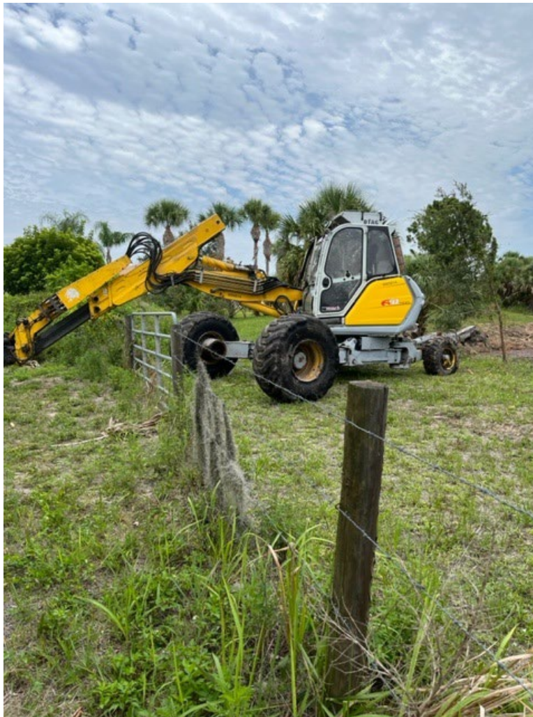
Photo of Menzi Muck, machine used to remove silt buildup within South Creek
